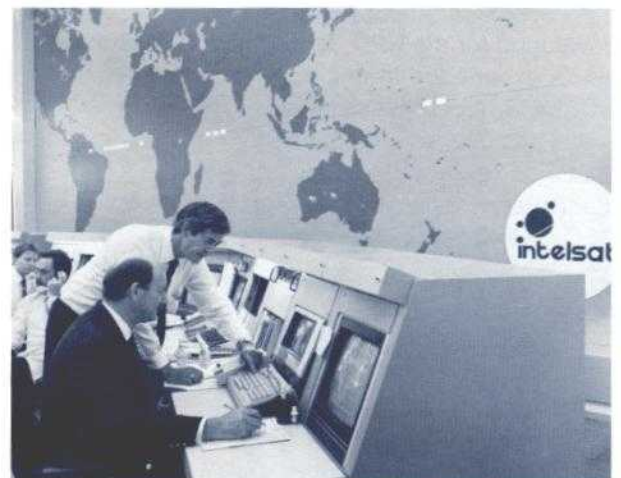
Figure 3. The INTELSAT Operations Center TDMA Facility provides centralized monitoring and control of TDMA satellite communications networks
