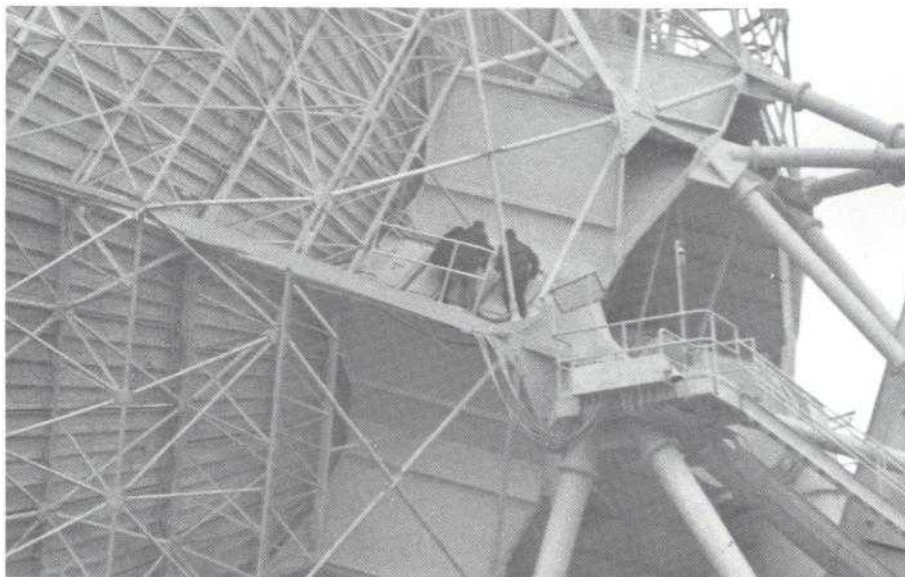
Andover technicians are almost lost to view as they work approximately 70 feet above the ground on the power panels of the 12-story-tall antenna structure.
